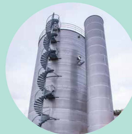
From the biogas facility at Saugbrugs.
